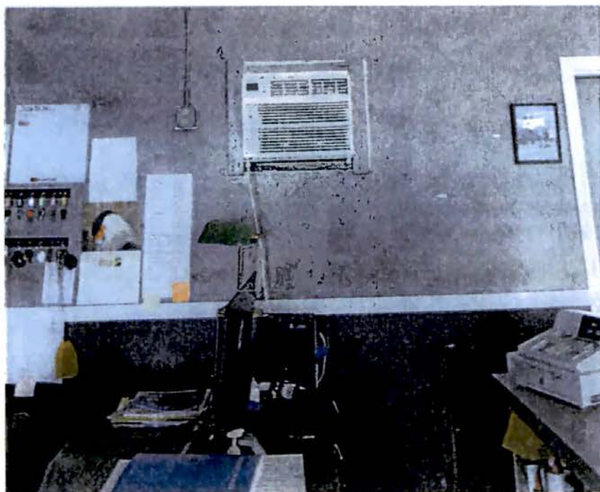
The office – wall installed AC unit
