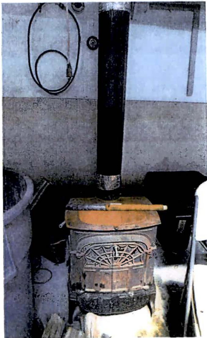
Maintenance garage – furnace (wood burning)
